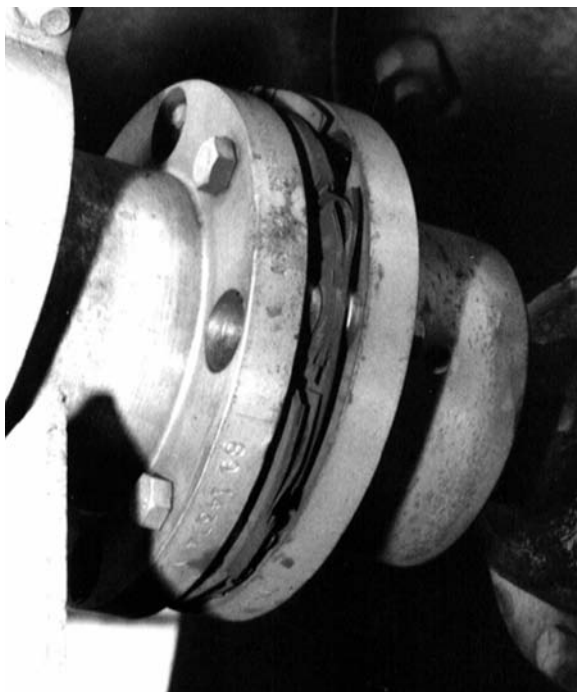
FIGURE 1.1 Disk coupling failure due to shaft misalignment.
